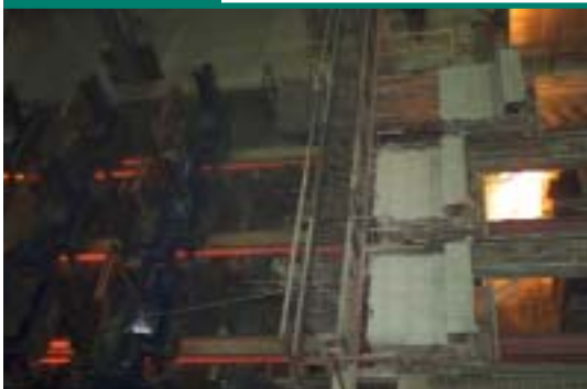
View of three beam blank strands exiting unbending and undergoing torch cutoff.
